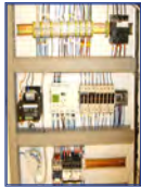
Electrical cabinet example
