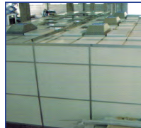
Rigid high walls in the mechanical industry
